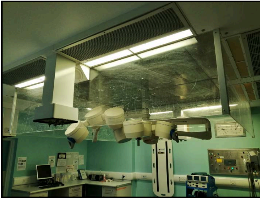
Figure 6: A typical orthopaedic theatre laminar flow HVAC system. Photo Dr J Major
